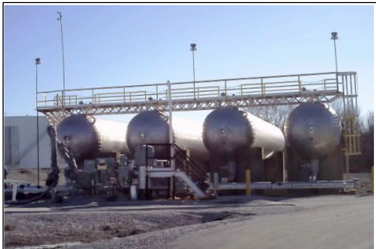
GHC biodiesel storage containers at Buckeye terminal
